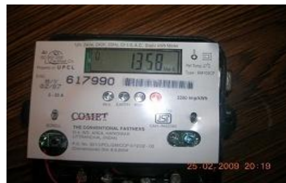
Fig. 2 Digital meter being used in Jammu & Kashmir
